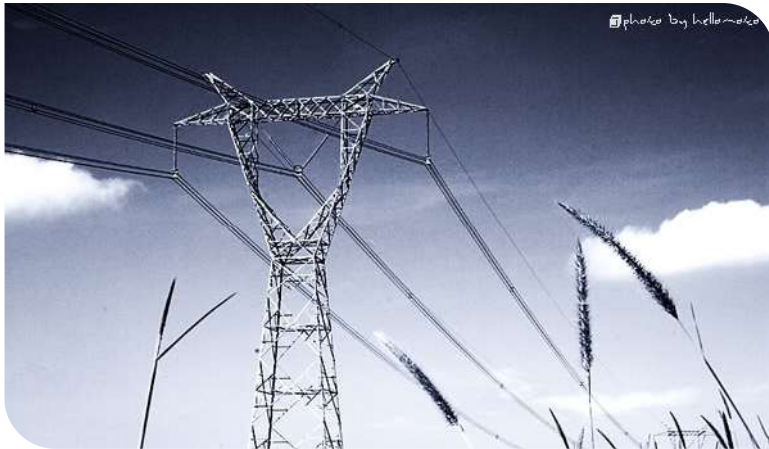
Cables for National 500KV overhead lines backborns 500KV.
